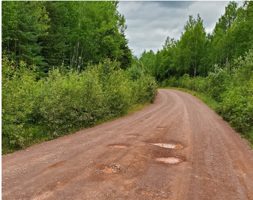
Figure 7: Potholes on an unpaved road surface
