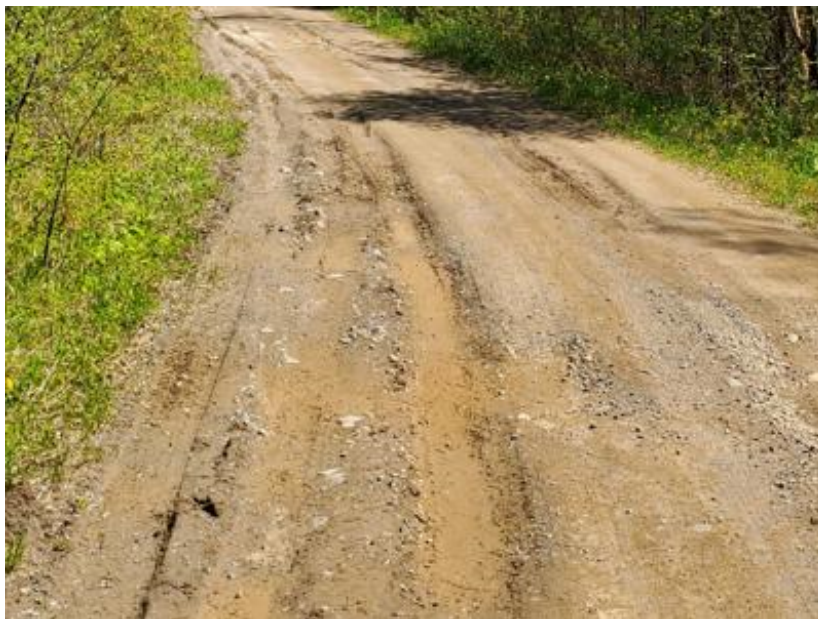
Figure 8: Rutting on an unpaved road surface
