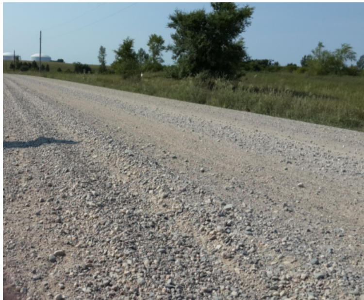
Figure 10: Loose aggregate on an unpaved road surface (From Jahren Charles 2015)
