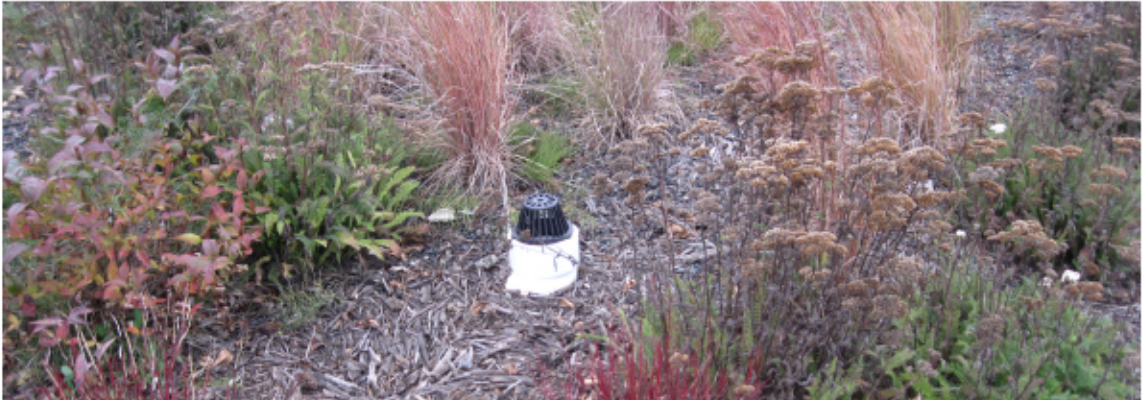
Figure 11. Drainpipe observation station (D&R LID)
