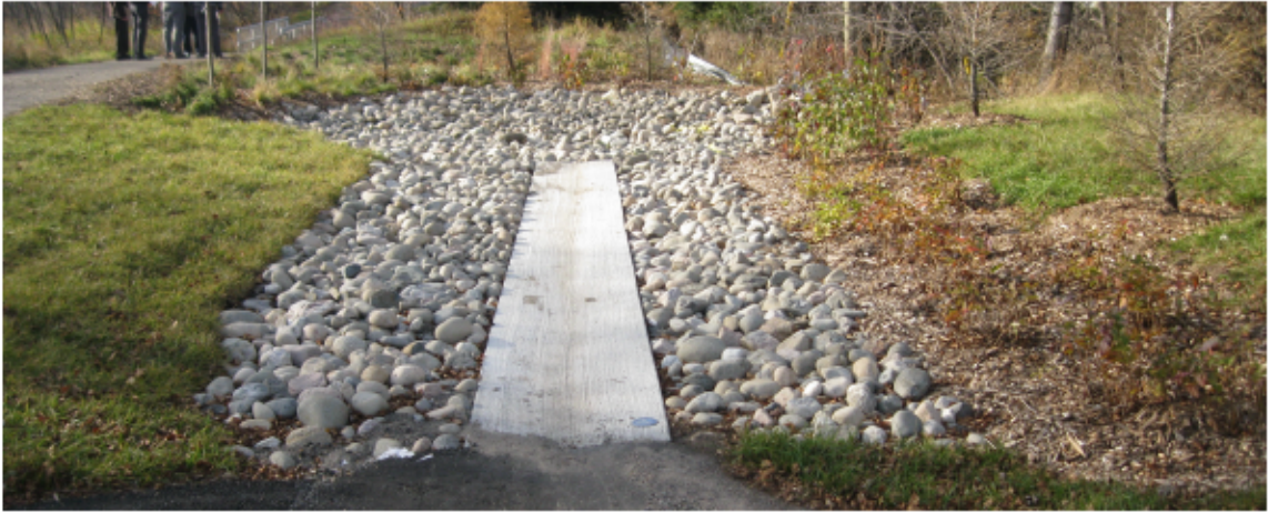
Figure 14. East LID entrance and pre-treatment (McVicar Creek LID)
