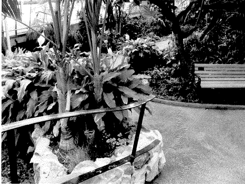
Figure A.6. A photograph of the stone retaining walls, cement walkway, and soil taken inside the Conservatory.
